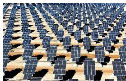
Solar Power plants
